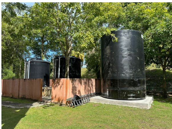
Water tanks photographed in the project progress report.
